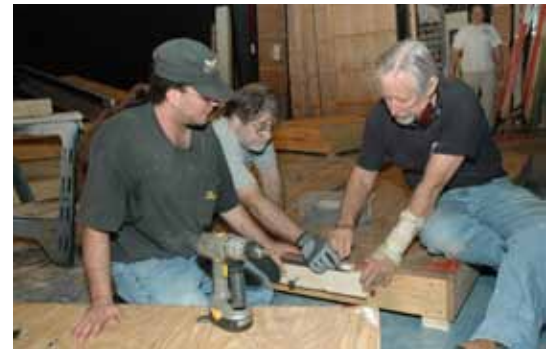
Never one to back away from hard work, Jason puts his carpentry skills to work helping Jim White (center), Michael Iles (right) and Adam Witko (standing) with the set construction for 1940s Radio Hour .
